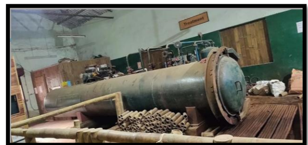
CCB (Copper Chrome Boron) Chemical Process Tank
