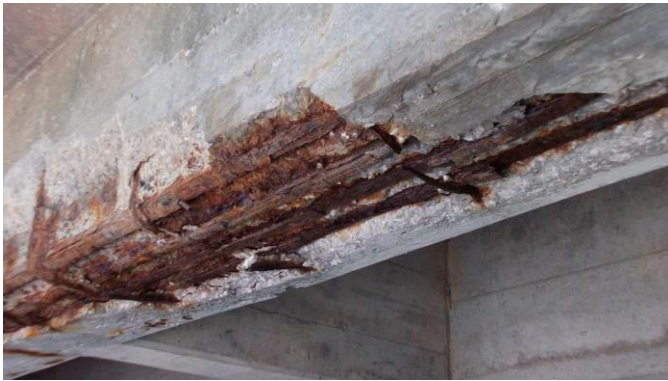
Fig.-2 Cracks in beams indicate corrosion of reinforcement
