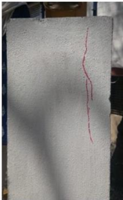
Figure 8 Formation of cracks in RS1
