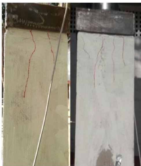
Figure 12 Crack pattern of RS3 formed at the top end
