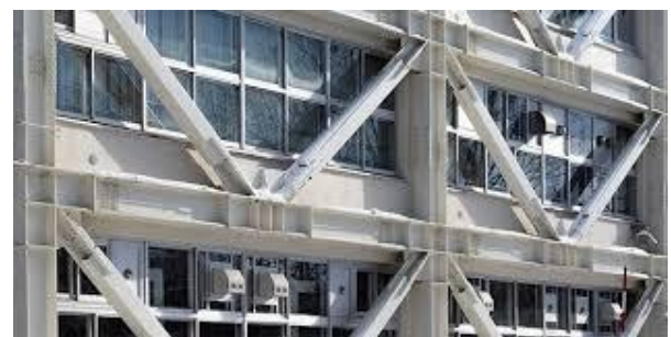
Figure 1: Seismic Dampers in Building
