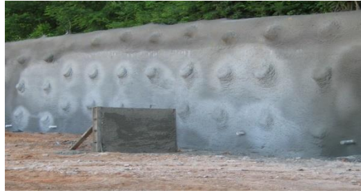
Fig3g: On-site shotcrete test panel curing is shown in the image. Thanks to Schnabel Engineering for the photo.. (Carlos A.Lazarte, 2015)
