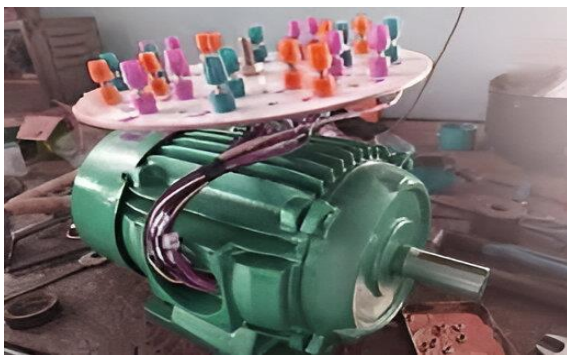
Fig - 7 : Inter-turn fault in stator with tapings exposed for testing
