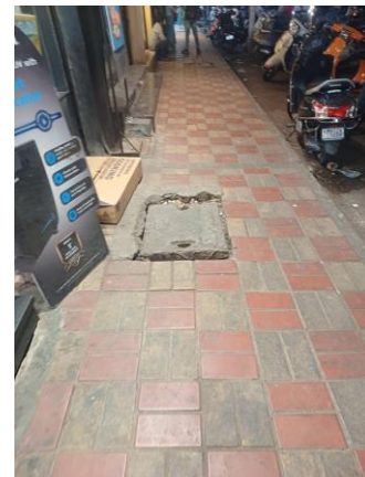
Fig 8: Sewer cover not in line with the footpath level on MG road. Source: Author
