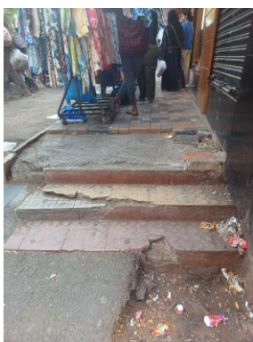
Fig 10: No ramps provided on footpath at MG road. Source - Author
