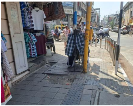
Fig 9: Missing tiles on footpath on Laxmi road. Source – Author
