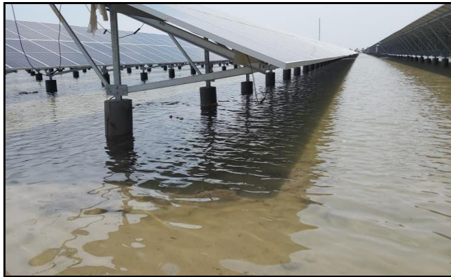
Fig -6: Flood Impact on Module Mounting Structure
