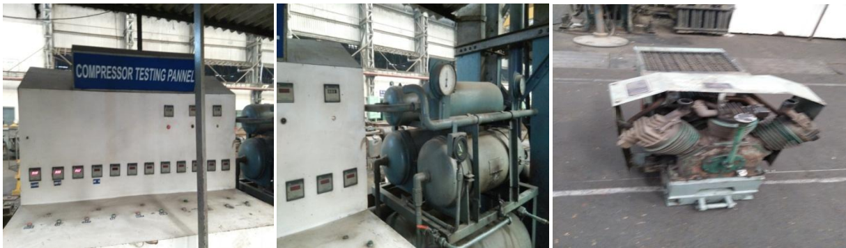
Fig.2.1 Compressor Testing Panel, Storage tank and Reciprocating air Compressor [18]
