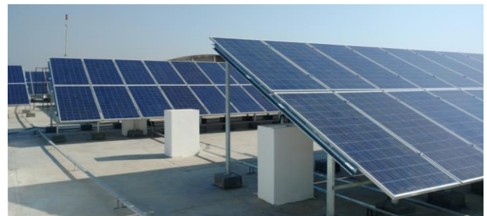
Figure 3: 100 kW P rooftop solar power plant at Poornima University
