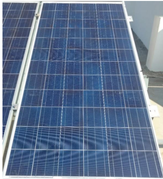
Figure 1. 300W solar module for experimental set up
