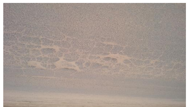
Fig 1:- Exsiting Pavement Condition
