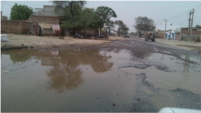
Fig. -3: Formation of ruts, cracks and pot holes and poor drainage system nearby Dhani Prem Nagar, Barwala Road.
