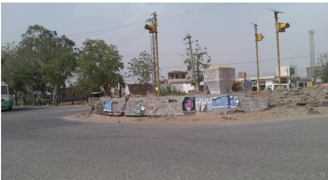
Fig. -4: Poor condition traffic lights, no pavement markings, bad condition of rotary island at Surewala Chowk, Barwala Road.
