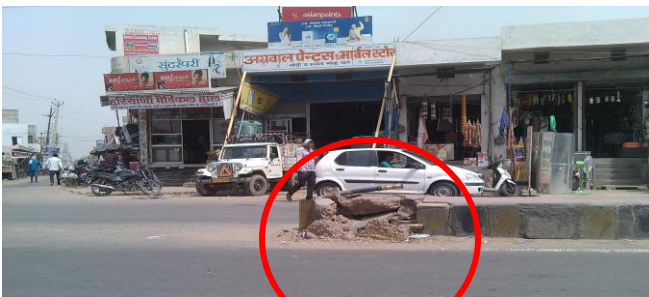
Fig. -6: Poor condition of delineators, reflectors and poor maintenance of traffic signs and symbols nearby Old bus stand, Barwala.
