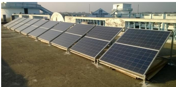
Figure 1: SPV Power Plant on the roof of JIS College of Engineering
