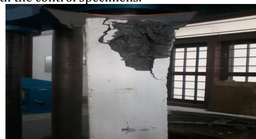
Fig. 10: failure pattern of column
