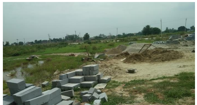
Fig.-5 Poor site management (Aerated Concrete Blocks stored in open)
