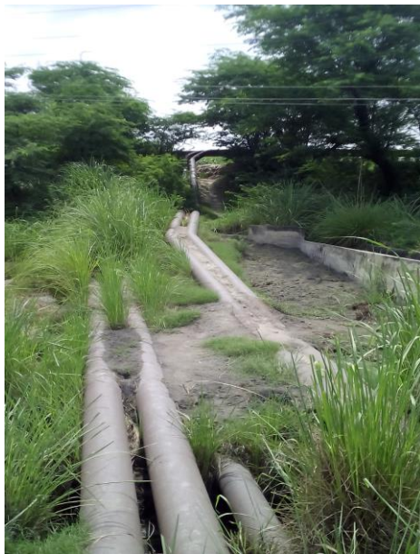
Figure 5. Pipelines carrying fly ash in the form of slurry..
