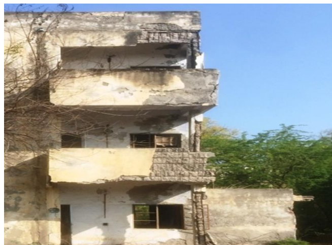
Figure 2:- Spalling of concrete and corroded reinforcement of building P-1003
