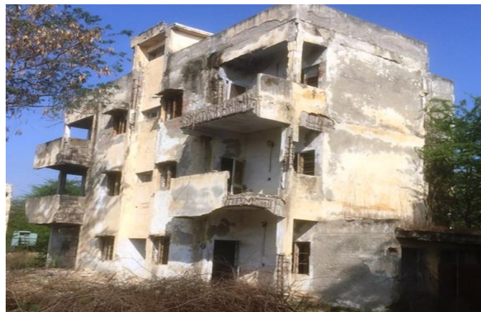
Figure 1:- Distressed condition of the building p-1001
