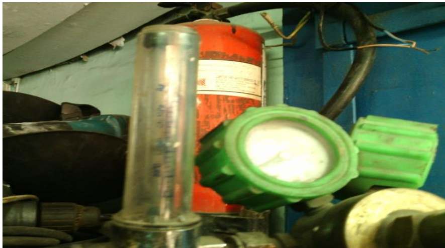
Figure 4: Argon Gas pressure gauge and gas flow regulator
