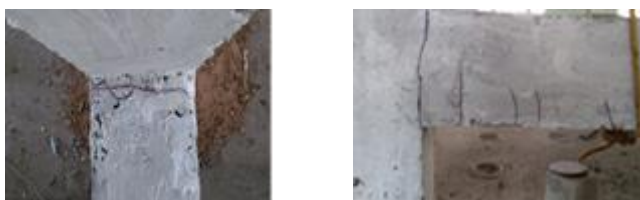
Fig.11. Crack pattern for specimen detailed as per is 456
