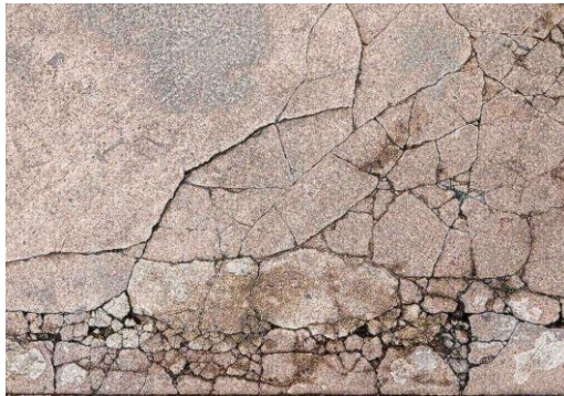
Fig -2: Non-Structural Cracks
