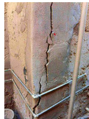
Fig -1: Structural Cracks
