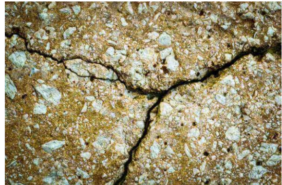
Fig -5: Wide Crack
