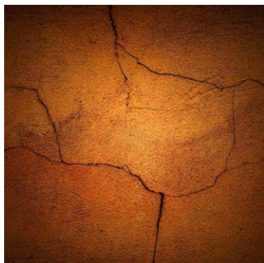
Fig -4: Medium Crack
