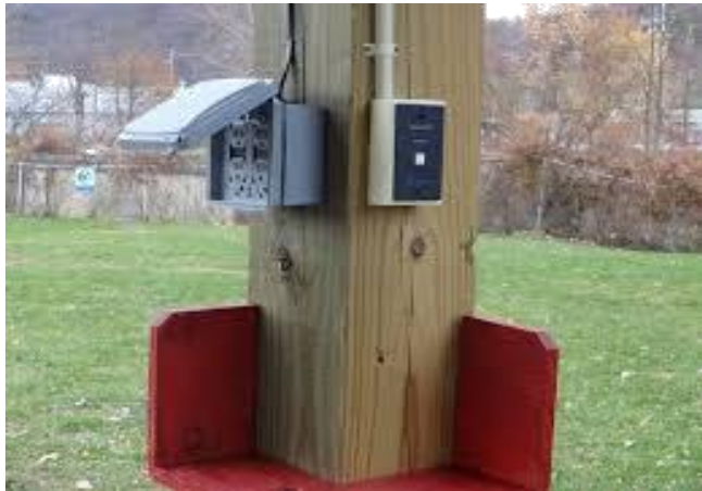
Fig 5. Mobile Charging Setup
