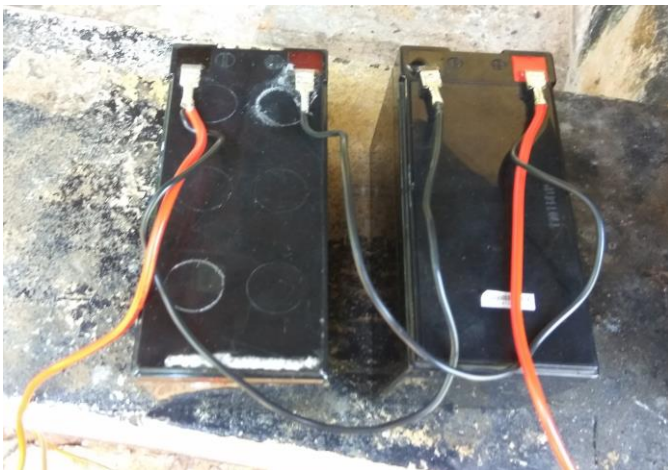
Fig -4: Battery in parallel connection
