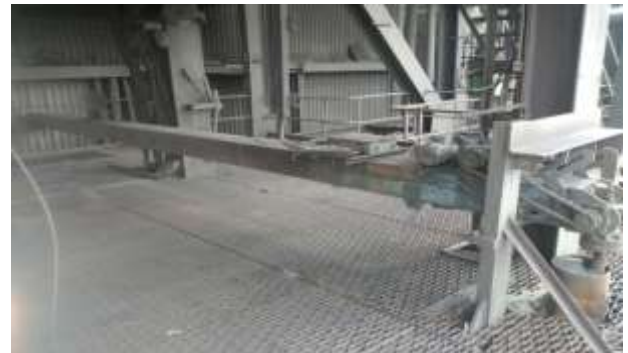
Fig 1.1: Actual image of LRSB inside the boiler
