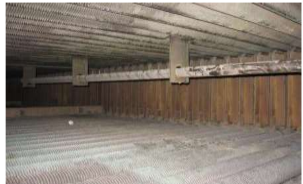
Fig 4.5: Actual image of lance tube with supports
