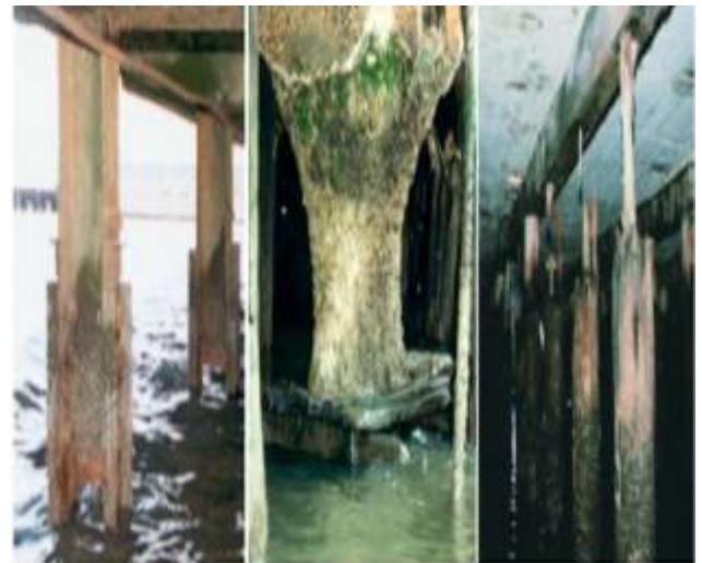
Fig-1: Degradation of Pile
