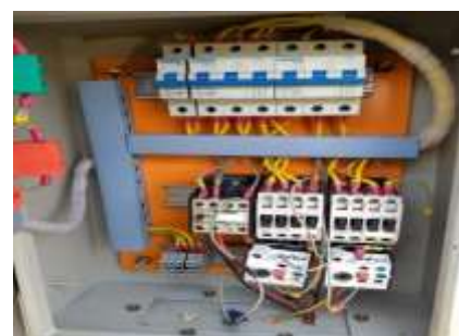
Fig-4: Control Panel
