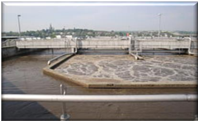
(Aeration tank of an activated sludge process at the wastewater treatment plant)
