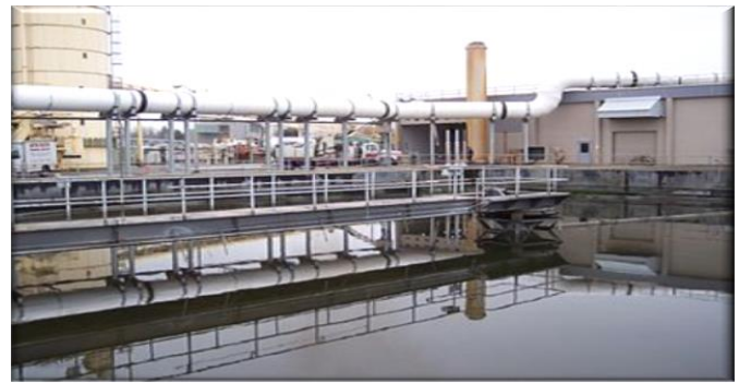
(Primary treatment tanks)
