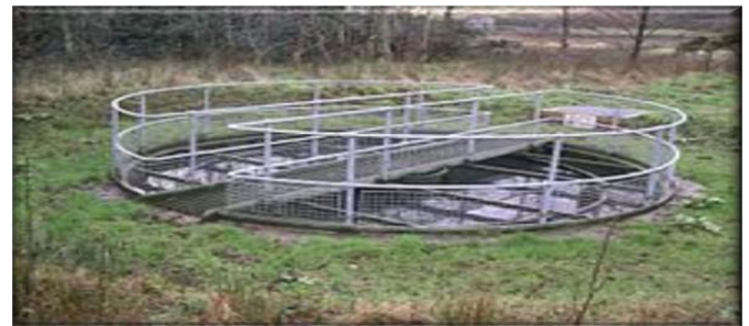
(Secondary clarifier at a rural treatment plant)
