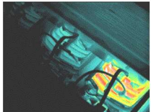
Above thermal image shows overheated windings on a step-down transformer, possibly caused by harmonics.
