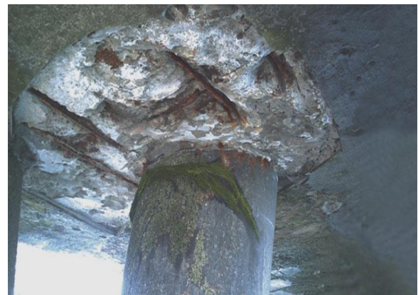
Fig -1: Deterioration of Concrete Structure
