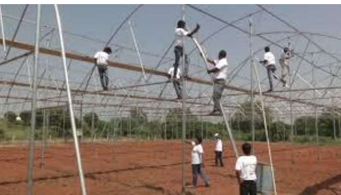
Fig-11: Method of Installation and removing of roof of polyhouse using labours
