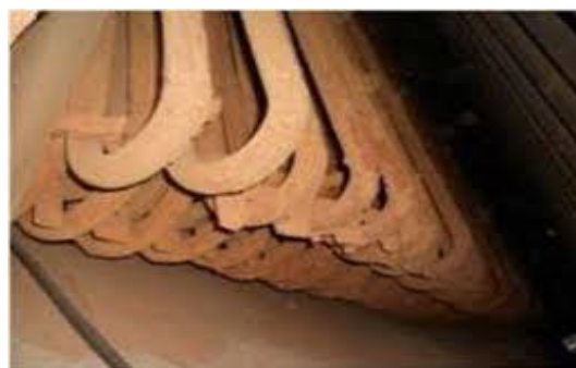
Fig 2 Soot Formation in Boiler Coils
