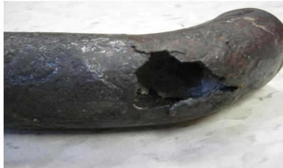
Fig 3 Boiler coil damage
