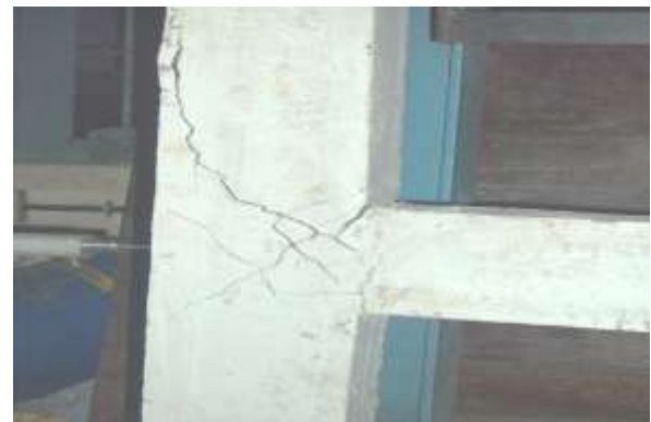
Fig.-8: Failure pattern of control specimen (CR)
