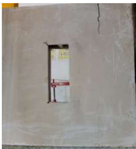
Fig-12: Crack pattern of panel with opening
