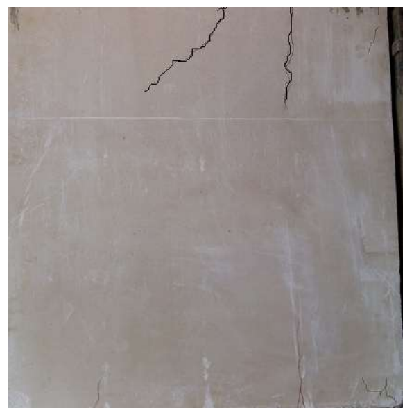
Fig-9: Crack pattern of panel without opening
