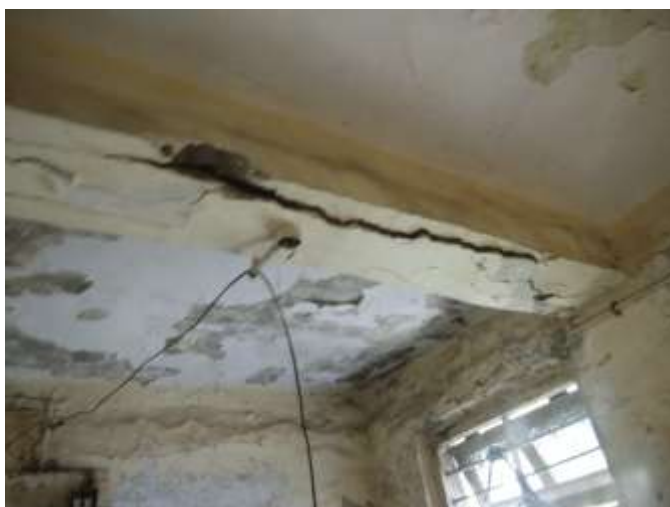
Fig -2: Cracks in beams
