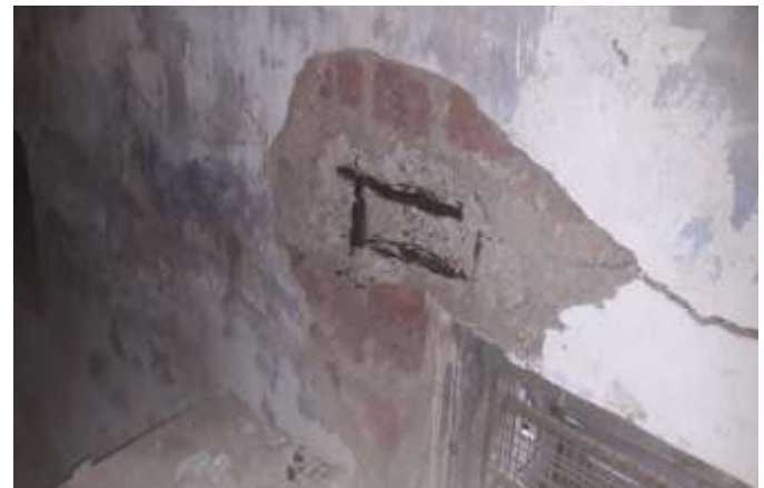
Fig -3: Exposed brickwork in walls
