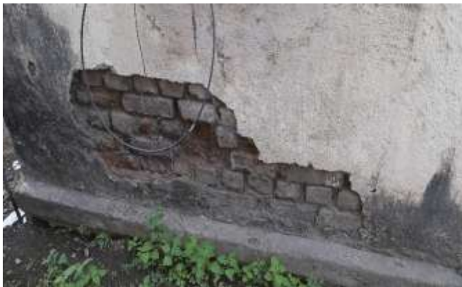
Fig -1: Exposed reinforcement in wall
