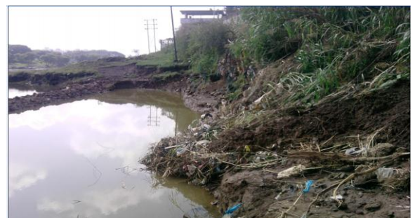
FIG 8- Bank erosion at Ordinance factory, Kirki, Pune
