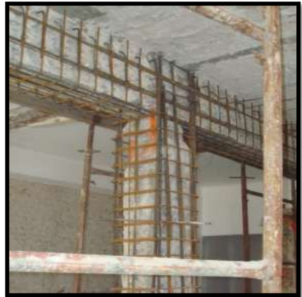
Figure -10: Depiction of RC Jacketing of Column as necessity for preventing the failure of columns in the building
