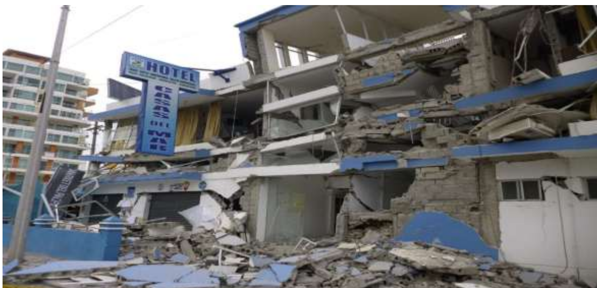
Fig 1: Building collapse due to lateral forces
