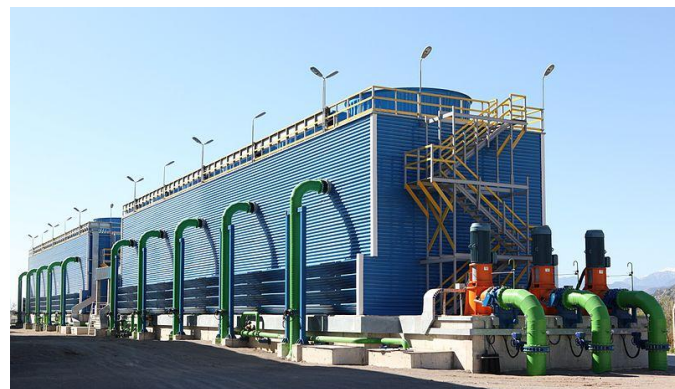
Fig. 1.2 Industrial Cooling Towers
