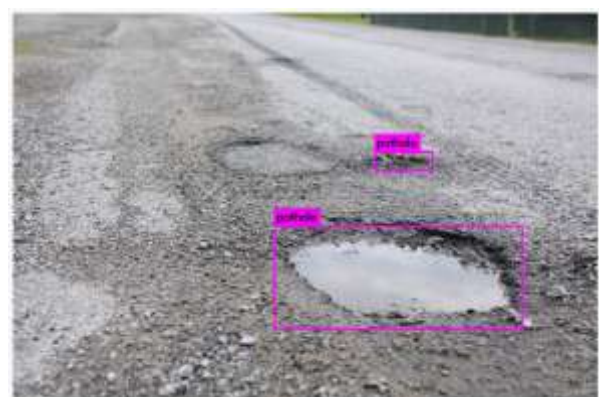
Fig -5: Pothole Detected using YOLOv3
