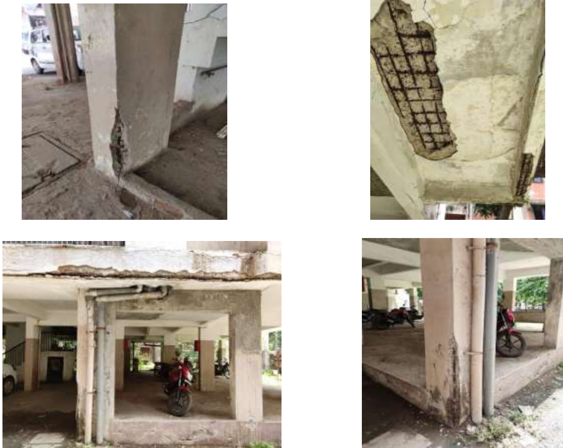
Figure 2 Deterioration Of Concrete In Slab, Beam, Column
