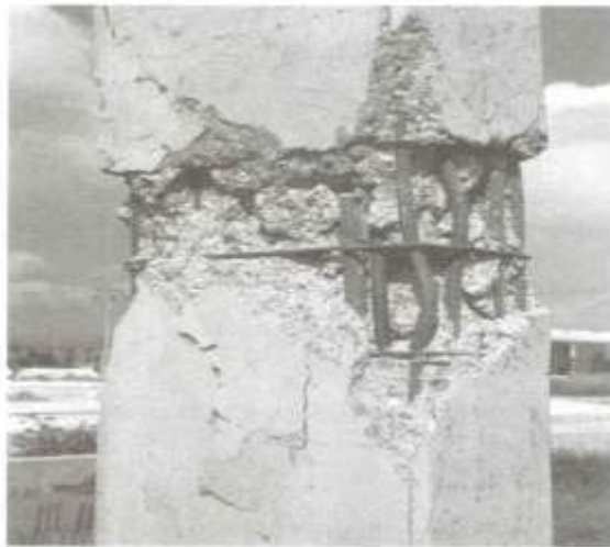
Fig -16: Close-up of poor column details
