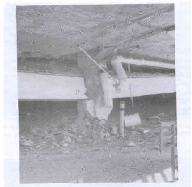
Fig - 15: Failure of poorly detailed precast concrete column
