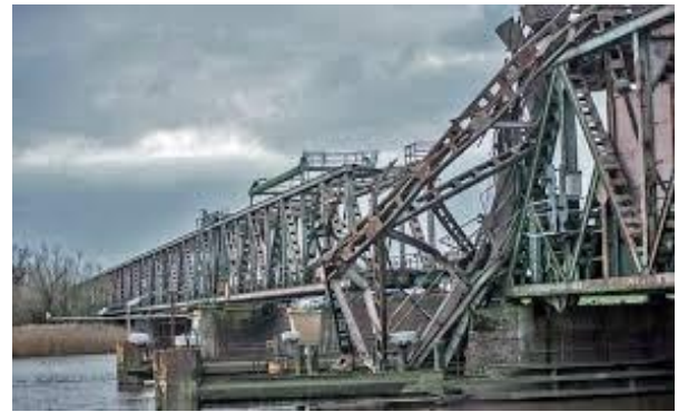
Fig -8: Collapsed Bridge
