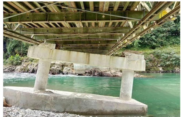
Fig -9: Damaged Bridge
