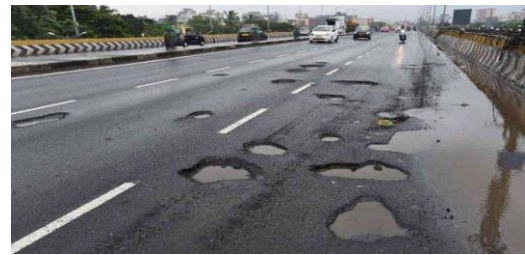
Figure -1.1: Pothole in roads
