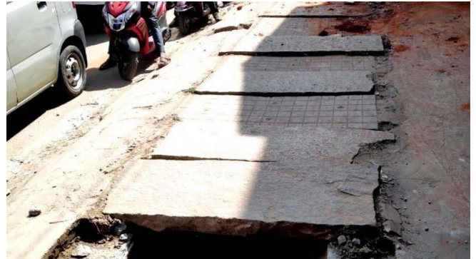
Fig - 1 Broken Drainage System
