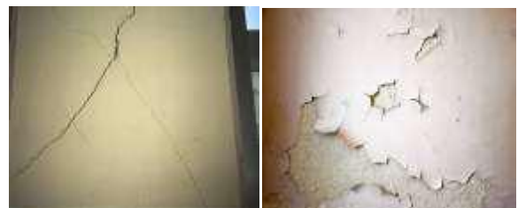
Photo -1: Visual Inspection of Cracks and Damages of Plaster in Building.
