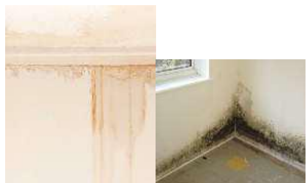
Photo -2: Visual Inspection of Leakage in Building.
