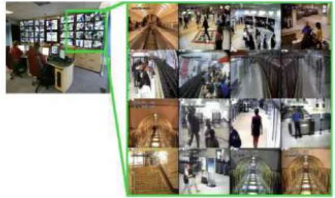
Figure 02: CCTV control room
