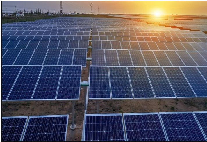
Fig -13: SOLAR POWER PLANT
