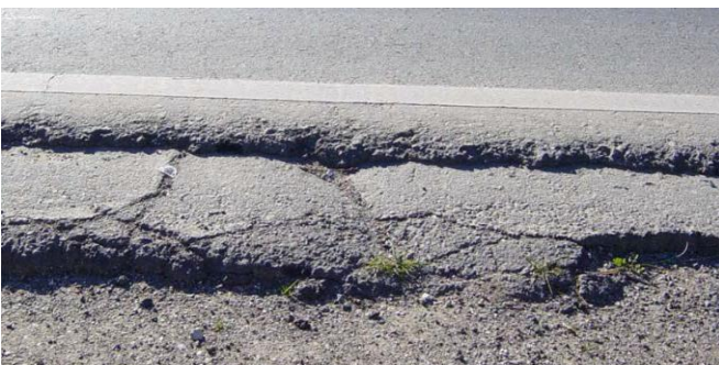
Figure 6. Edge cracking on road
