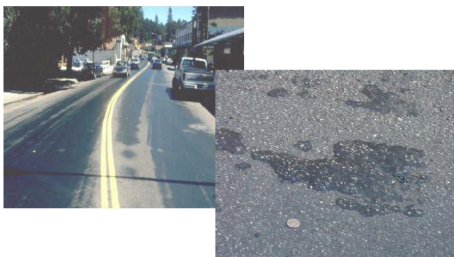
Figure 24. Bleeding on road
