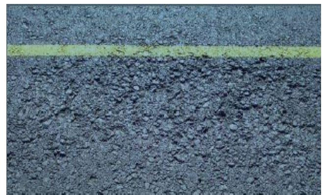
Figure 20. Segregation of Coarse Aggregate
