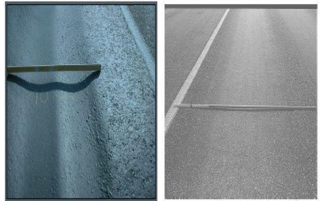
Figure 7. Rutting on road
