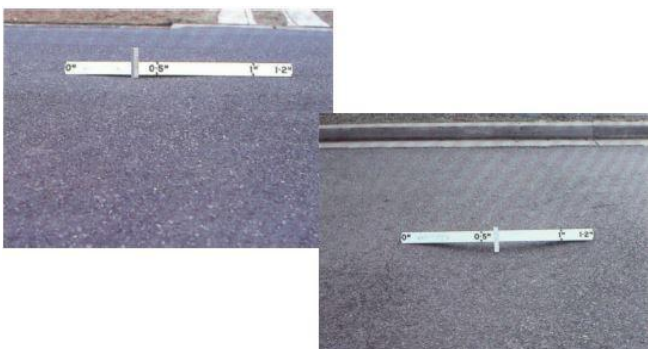
Figure 12. Depression on road
