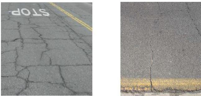
Figure 5. Block cracking on road
