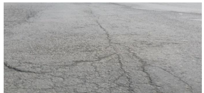
Figure 3. Longitudinal cracking on road
