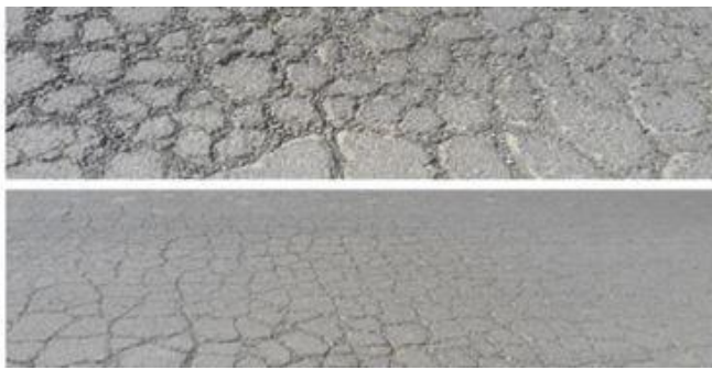
Figure 4. Fatigue cracking on road
