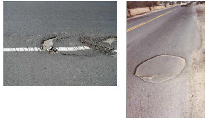
Figure 14. Delamination on road
