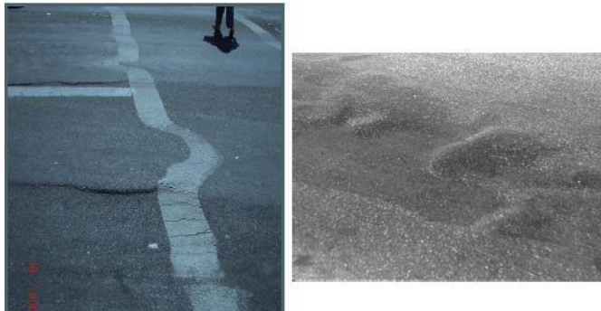
Figure 11. Shoving on road
