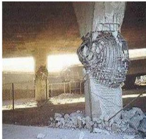
Fig – 6: Column Shear Failure during Bhuj
