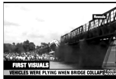
Fig -1: Bridge Failure (Media Information)
