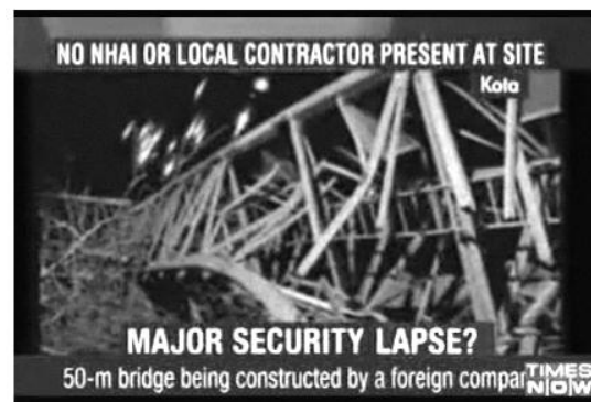
Fig - 2: Bridge Failure (Media Information)
