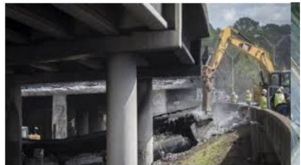
Fig – 8: Collapse of Bridge in I-85
