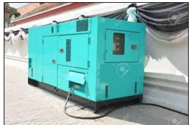
Fig-1: Emergency Diesel Generator (EDG) with canopy made up of sheet metal
