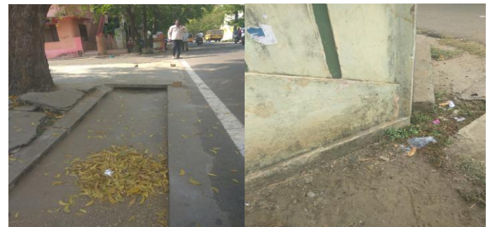
Fig -3: Damaged storm water drain in Bharatiyar street, Karaikal
